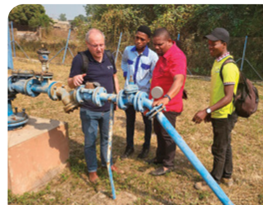
Christophe Leger, Deputy Managing Director of VERGNET HYDRO, and Dominique Da Cruz, Managing Director of OMILAYÉ, accompanied by OMILAYÉ employees, can be seen taking stock of some of the DWSs now managed by OMILAYÉ.
